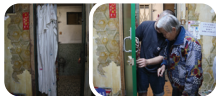
長者住所的屋內環境只靠布幔遮蓋，工程人員為長者裝上新的木門。 Contractor helps an older person to install a new wooden door to replace the curtain originally used to cover the doorless entrance.
