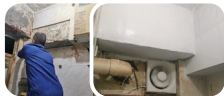
長者住所浴室經工程人員維修後環境大大改善了。 The bathroom environment for an older person has been largely improved after home improvement work by the contractor.
